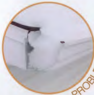
ICE BUILD-UP DEFORMATION
