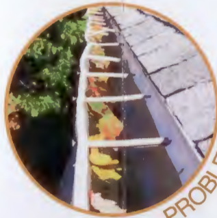
WARPED RAIN GUTTERS
